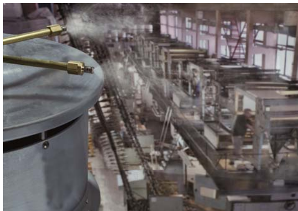
High level high pressure spray providing cooling within a Printing Hall
