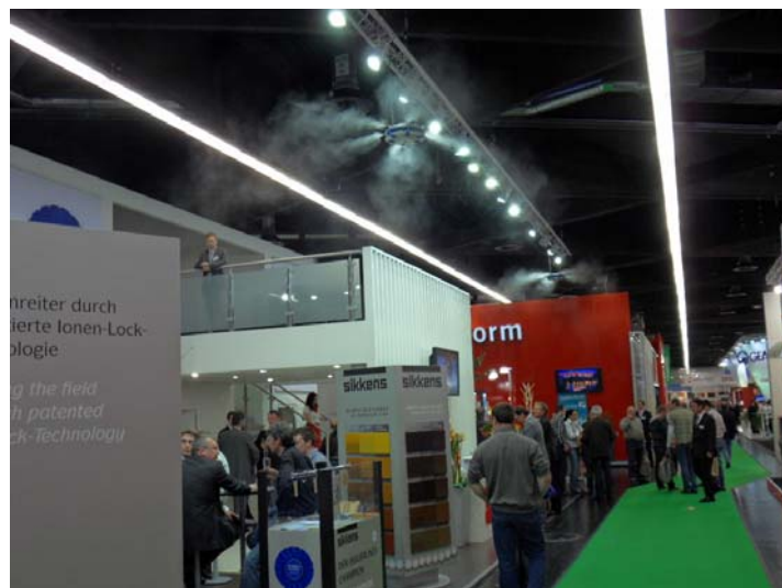
Exhibition hall cooling
